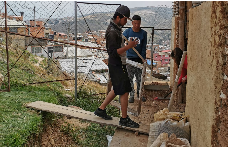
Residents of Cazuca building structures to create a resilient community against the pandemic.
